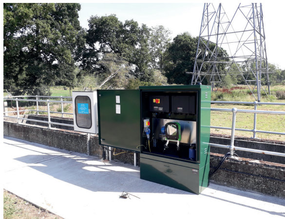
ESNET Kiosk at Wastewater Treatment Works
