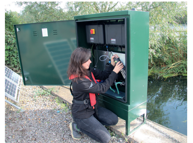
ESNET Water Quality Monitoring System
