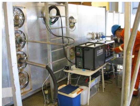
Figure 2. Sampling of biogenic CO 2 at the waste incineration plant (Næstved Waste Incineration Plant) during the field test.
