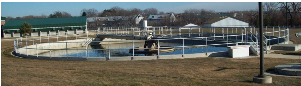
The City of Watertown Wastewater Treatment Plant Settling Tanks
