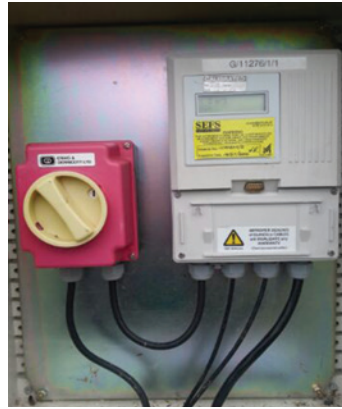
Whatever meter you fix you have to maintain. The pictured meter worked for a number of years but without the correct maintenance will fail
