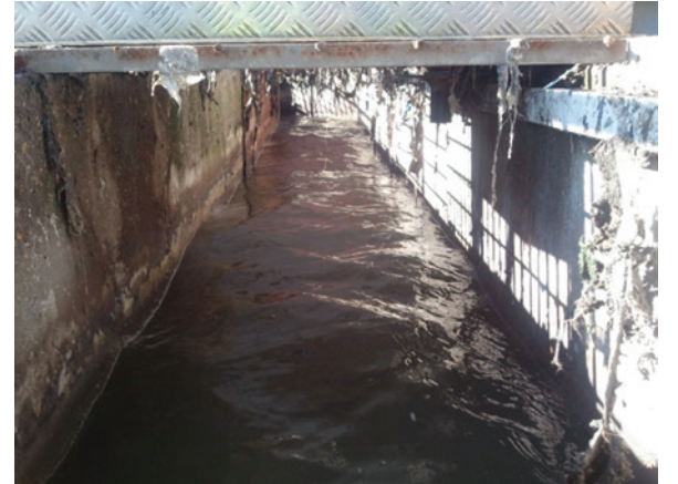
Choosing the right meter for the right place is essential. The flow meter installed in this channel (see if you can spot it) can't possibly work correctly considering the conditions its expected to work in
