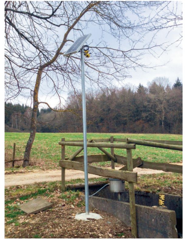
Since no power connection is available at this location, the measured values are recorded every hour by a PLICSMOBILE T81 with accumulator and solar panel and forwarded to VEGA Inventory System.
