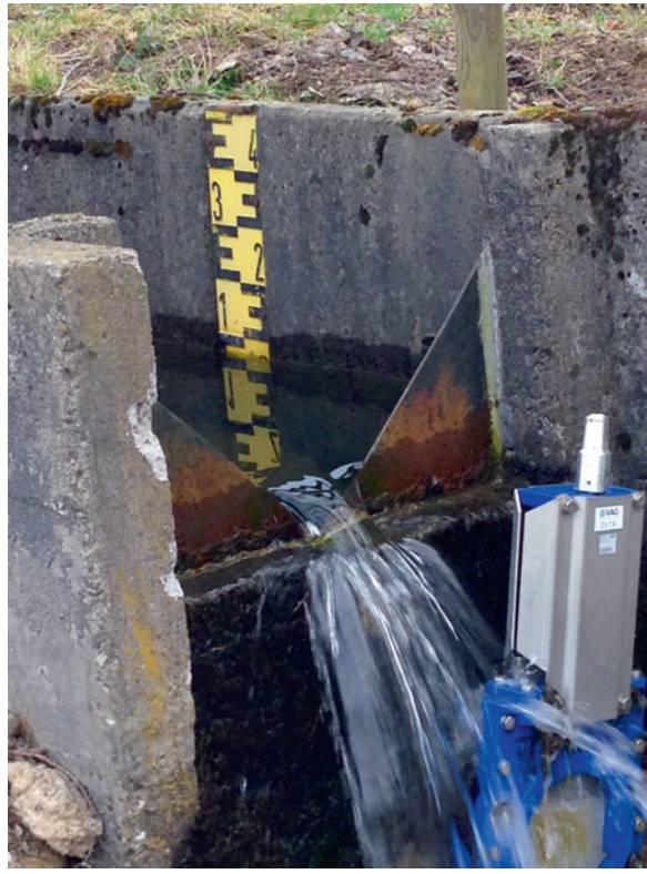
The flow in the open channel is measured by means of a V-weir at the inlet. VEGABAR 86, an immersible pressure transmitter for level measurement in wells, basins and open vessels, is used here.
