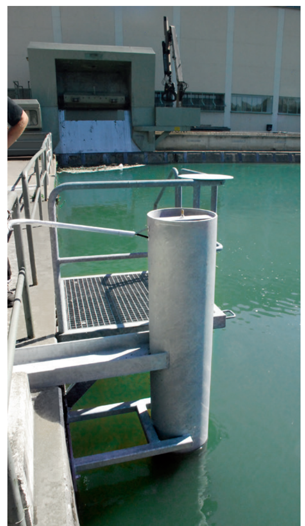
Flotsam is no problem here: A sturdy pipe provides additional mechanical protection for the level measurement system.
