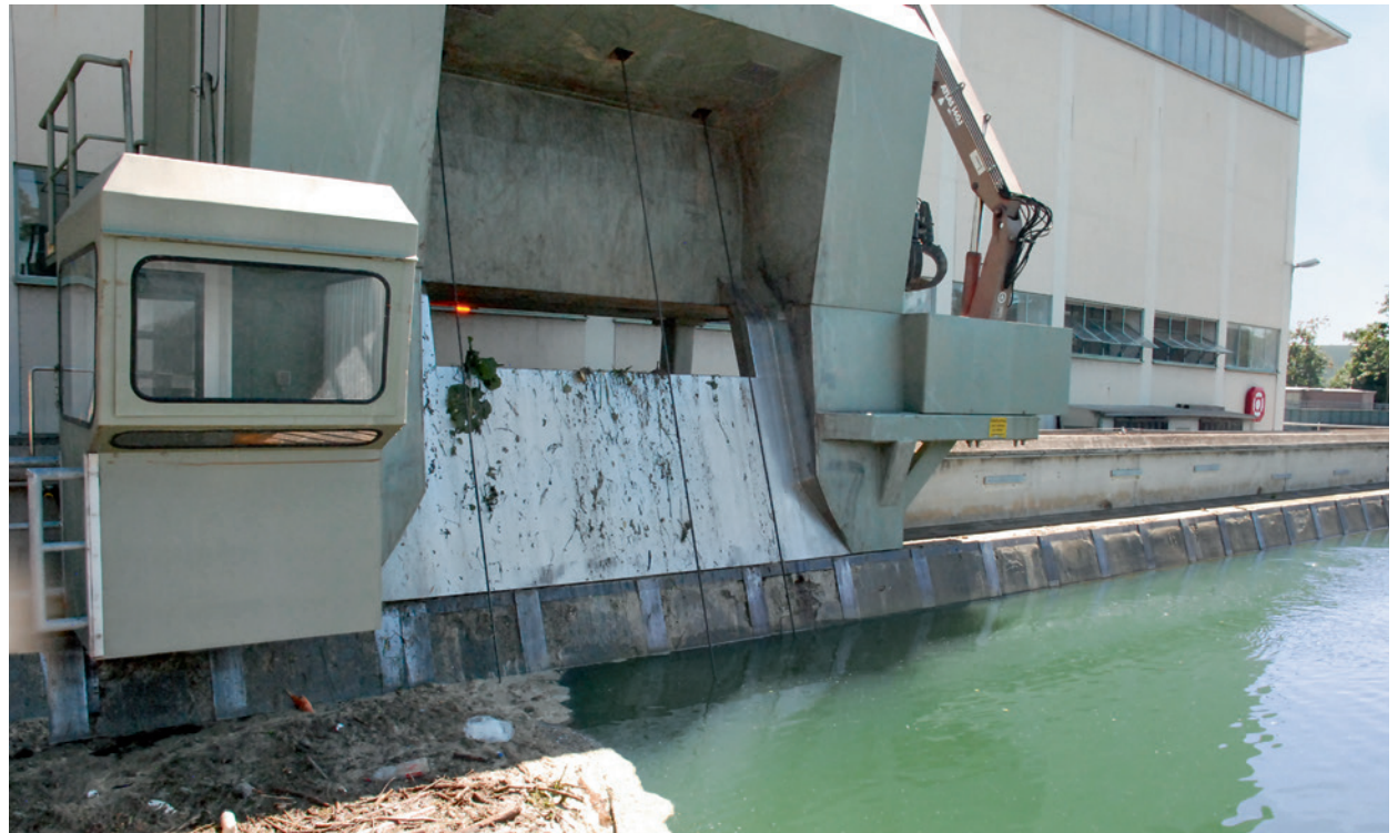
Located a short distance the inlet structure, a VEGAWELL 52 suspension pressure transmitter provides redundancy with a second measurement, complementing that of VEGAPULS 64.
