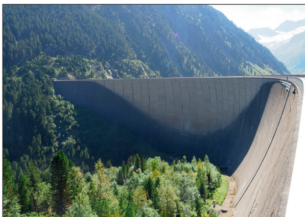
The doubly curved arch gravity dam is 131 meters high; one million cubic meters of concrete were used in its construction.
