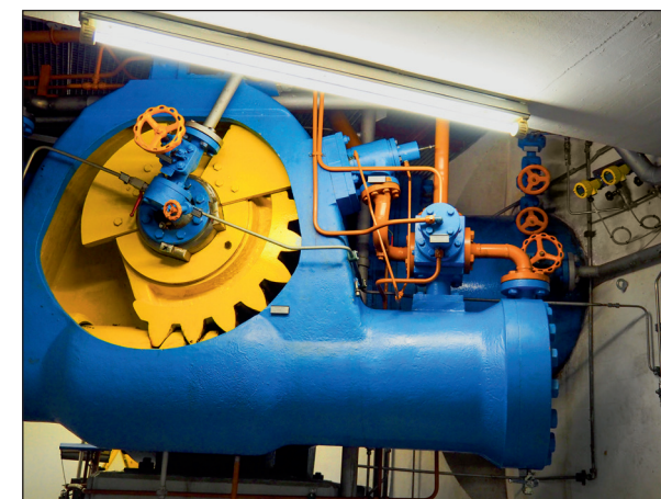
There are numerous sensors from VEGA not only in the dam itself, but also in the Roßhag power station. Compared to this huge shut-off valve, the two sensors are tiny.
