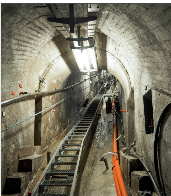
Technicians regularly walk through and inspect the numerous passageways inside the dam. In addition to the visual checks that are part of the routine maintenance, there are many measuring points with sensors whose values are electronically transmitted.
