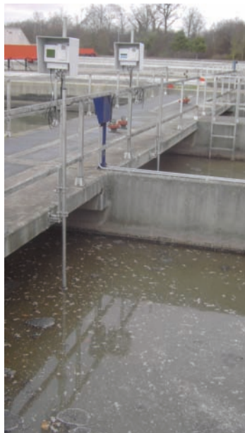
Fig. 5: Simple installation thanks to variable fitting systems. The best measuring point depends on the hopper design and must be determined by carrying out comparative measurements.
