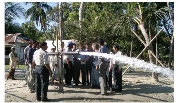
Pumping the deep aquifer at 700 gallons a minute to test the aquifer properties
