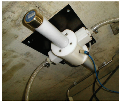
Figure 1: spectro::lyser™ in bypass installation.
