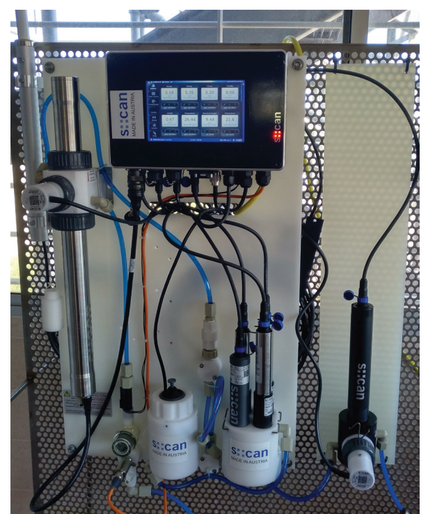
A micro::station monitoring the drinking water quality
