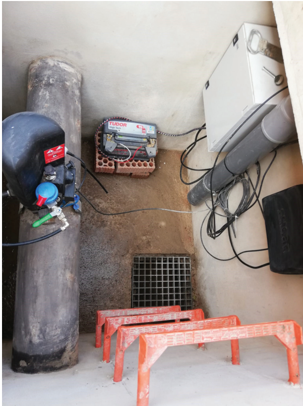
A pipe::scan installation in a manhole, on the left the pipe::scan, on the right the terminal control unit
