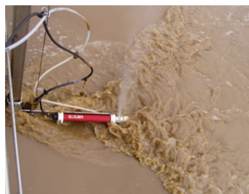
Figure 2: s::can nitro::lyser™ installed at Vienna's Main Sewage Treatment Plant
