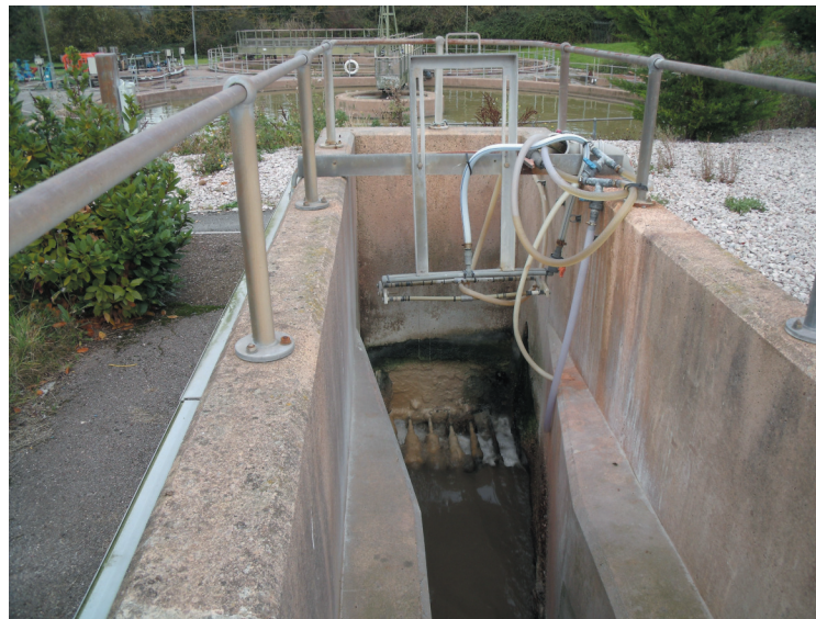
Figure 1: Partech TurbiTech 2000LS units were installed at the front end of the works
