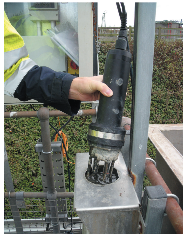
Figure 2: Partech Turbi-Tech 2000LS positioned at the BAFF splitter tank
