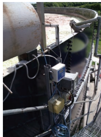
Figure 1: On the aeration tank (AT3), Partech's OxyGuard DO monitor is employed to measure the level of dissolved oxygen and ensure that the treatment process maintains the correct levels for effective treatment.
