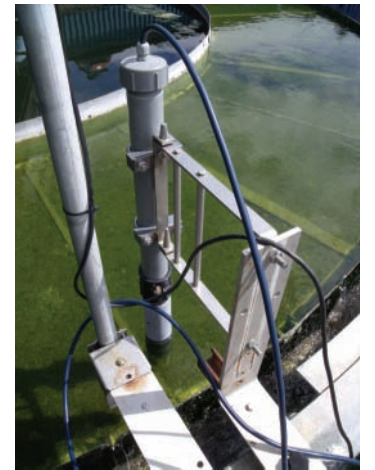
Figure 2: The treated effluent from AT3 tank passes via a settlement tank into the lockertex filter system, which is equipped with a Partech Turbi-Tech 2000LS turbidity monitoring system prior to point of discharge.
