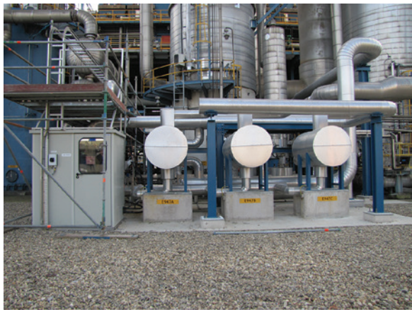
Analyser shelter with 3 heat exchangers
