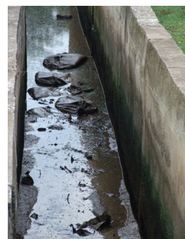
Figure 2: Open sewage pipe in Tra Noc Industrial Zone (IEEM, AKIZ-Project, sponsored by Federal Ministry of Education and Research)
