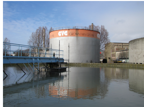
Holding Buffer Tank
