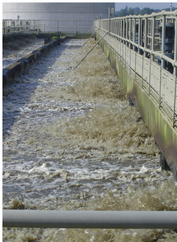
Aeration can be responsible for up two thirds of a treatment plant's total costs
