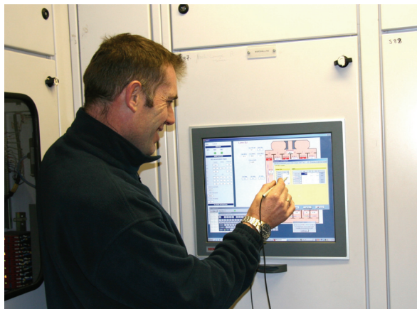
Matt Crowhurst with the W.T.O.S at Bournemouth WwTW
