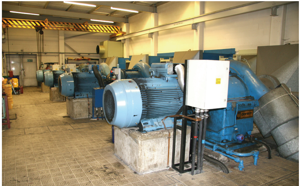
Electric blowers provide aeration for sewage treatment
