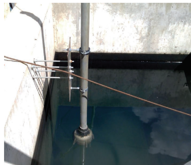
Sonatax sc probe over sludge collection hopper.
