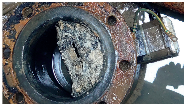
Photo above illustrates detritus build-up inside a magmeter. Clearly, this magmeter was in need of a better cleaning regime.
