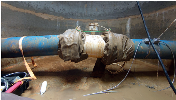
Photo showing a poorly installed magmeter. Note, the crooked pipework.
