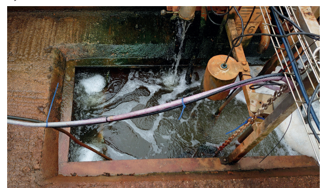
This photo shows a completely over-whelmed and drowned out V notch weir as a result of the factory expansion and subsequent increased flow rates, with no consideration for the flow measurement system. It also illustrates an over-cluttered chamber full of sample probes and pumps. As a result, it failed its MCERTS audit and had to be replaced.
