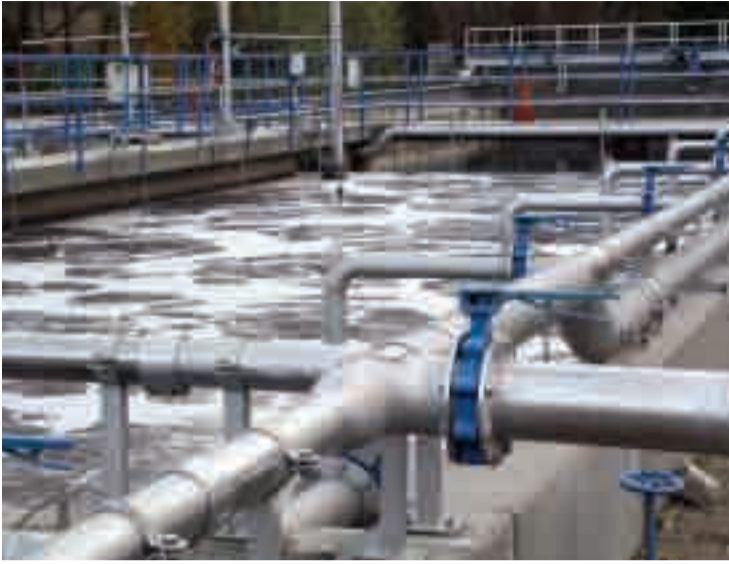
Aeration basin of a municipal water treatment plant today
