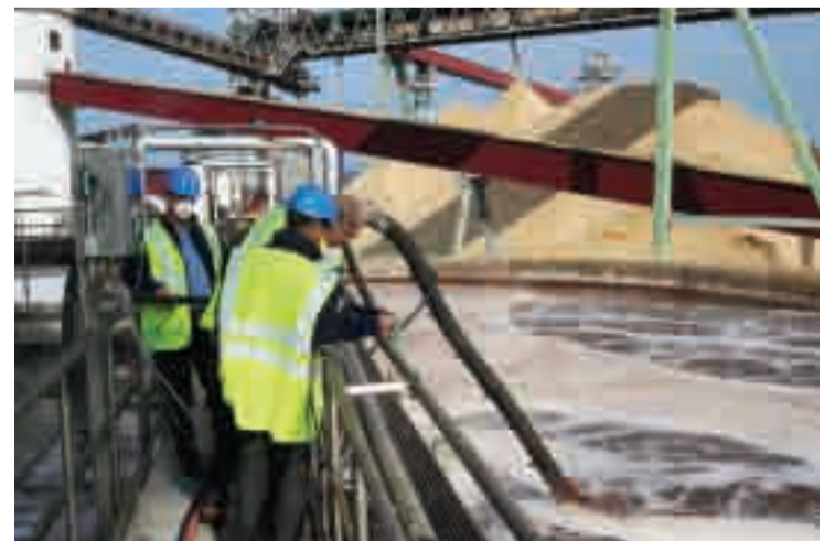
Aeration basin of an industrial water treatment plant today
