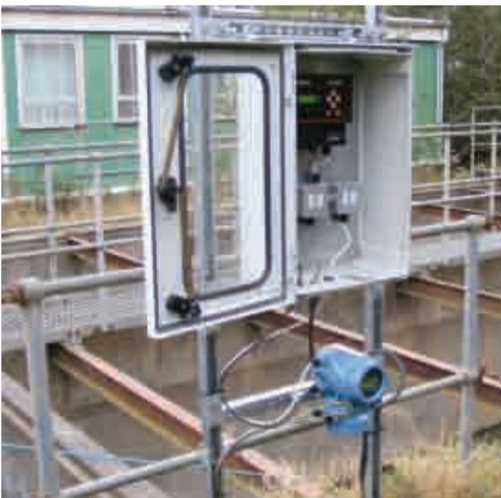
Waste management services company Waste Recycling Group is auditing its landfill sites and bringing their flow measurement up to MCERTS standards. The company has commissioned Emerson Process Management's Mobrey Measurement Division to provide a complete MCERTS compliant flow measurement package for each site, consisting of a self-calibrating Rosemount magmeter and a combined controller and data logging unit, the Mobrey MCULOG.
