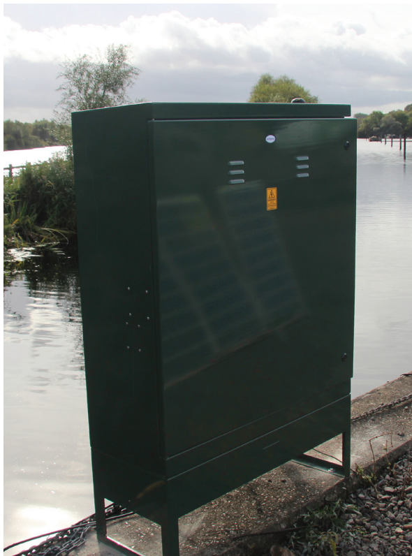
Water Quality Monitoring Station
