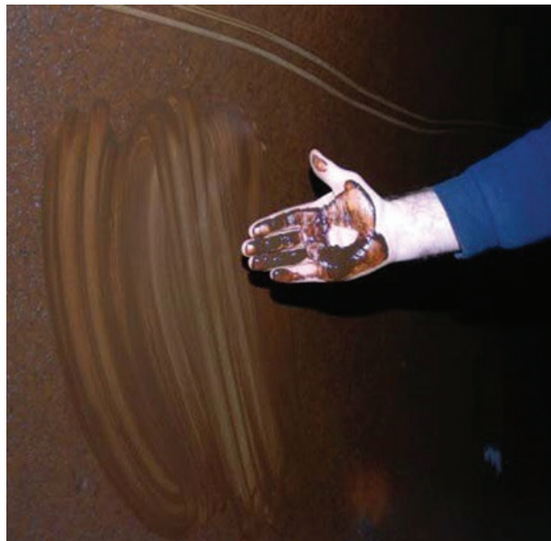
Biofilm on Water Mains, the Cause of Turbidity
