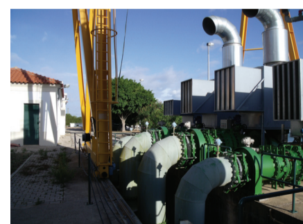
Fig. 2 KSB SNW Series pumps for raw water intake at Tavira.
