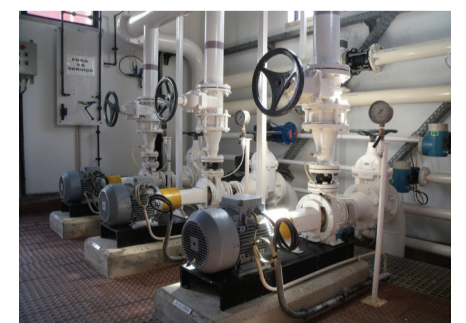
Fig. 3 Horizontal installed KSB Etachrom pumps for treated water distribution.
