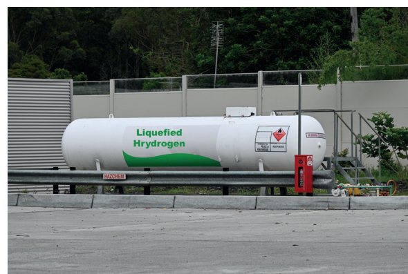
Liquid hydrogen storage
