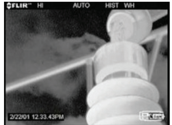
During their first FLIR training course, SSEPD identified a leak on a recently installed high-voltage circuit breaker.
