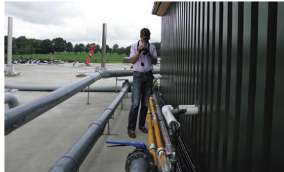
Explosion protected areas can be investigated with the FLIR GF320 from a safe distance.
