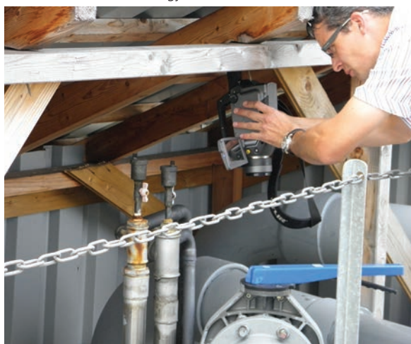
Engineer Ibeling van Lessen looking for gas leaks, which is possible from a safe distance and unusual angles using the FLIR GF320.
