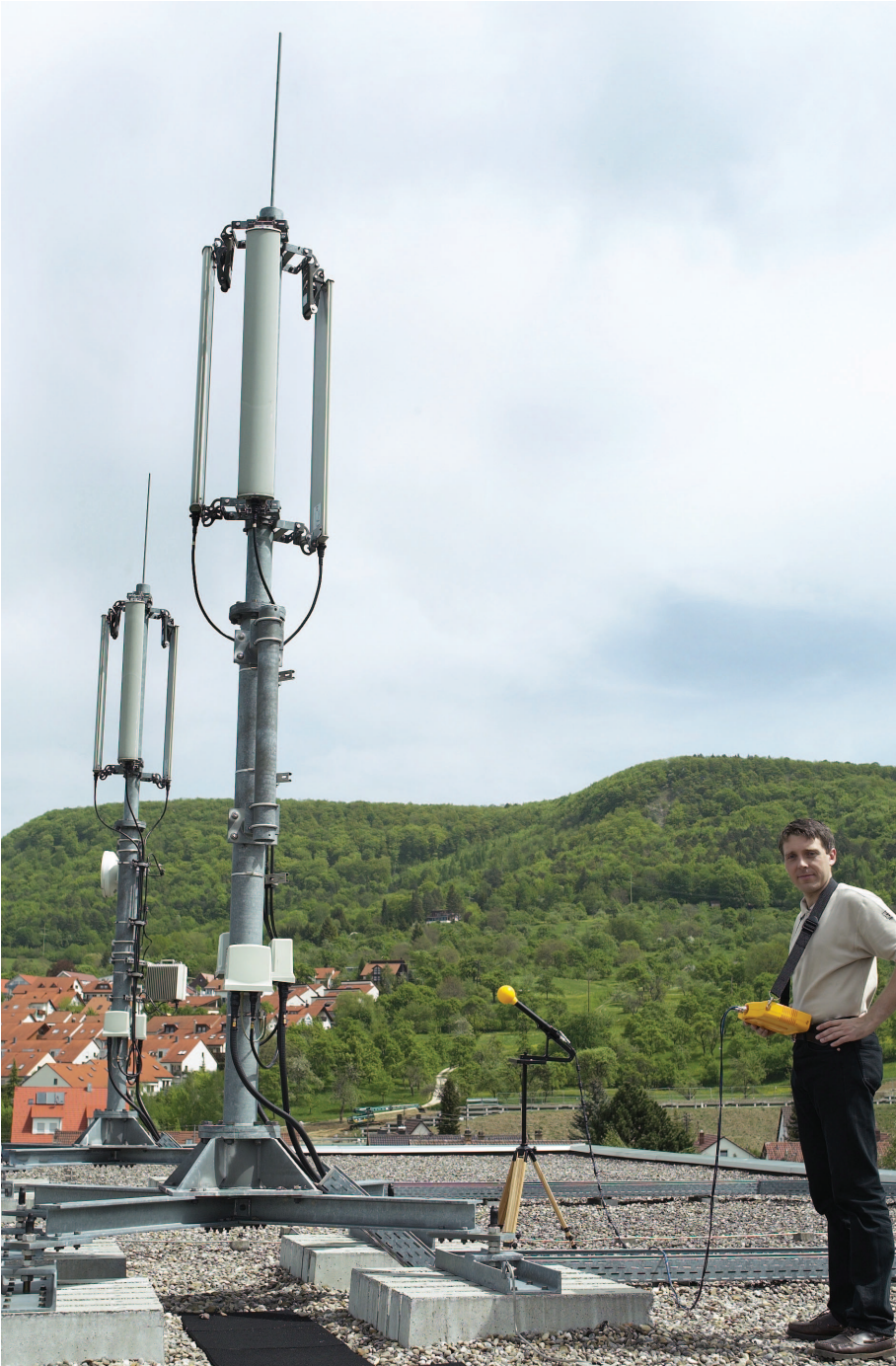
Fig. 2: Rooftop comparison measurement. The probe can also be fitted to a tripod for making precision measurements.
