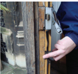
Figure 5: Seal missing on external door
