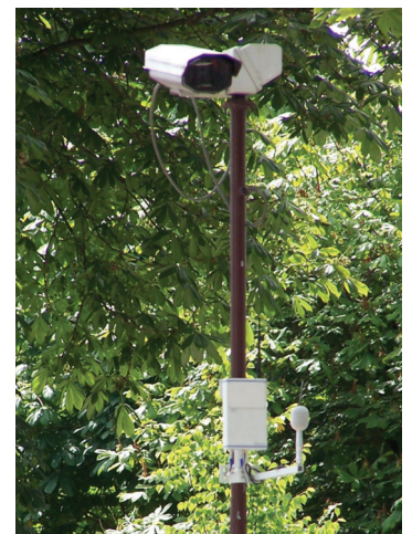
Figure 2: On-site implementation of OPER@ stations on video-surveillance poles
