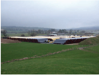
When completed, the pipeline will have the capacity to carry 20% of the UK's Natural Gas supply
