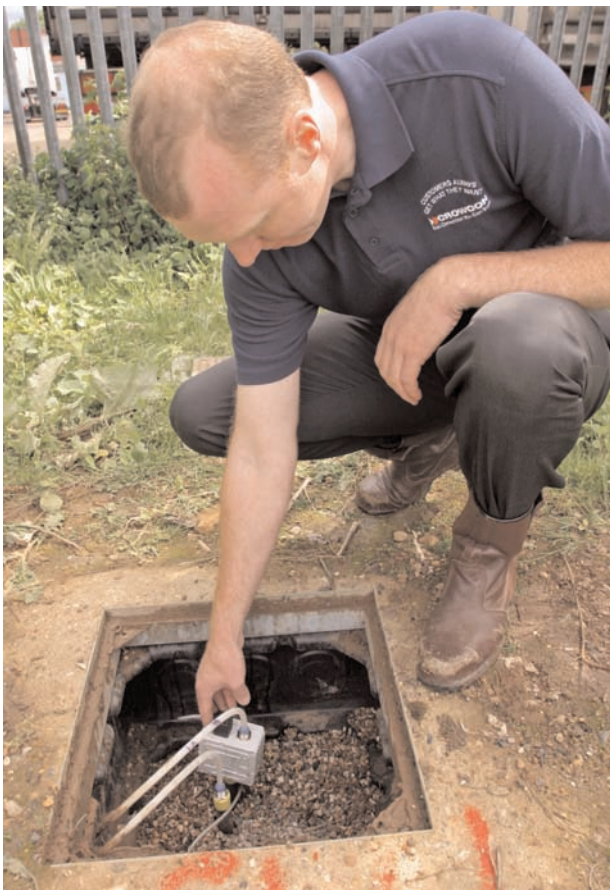
A borehole monitoring point with gas sampling tubes and a pressure transducer
