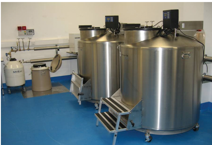
A typical cryoroom facility at John Radcliffe Hospital
