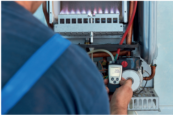
Flue gas testing on a boiler
