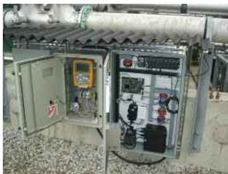
Static field gas analyser and (right) field server unit logs and transmits data
