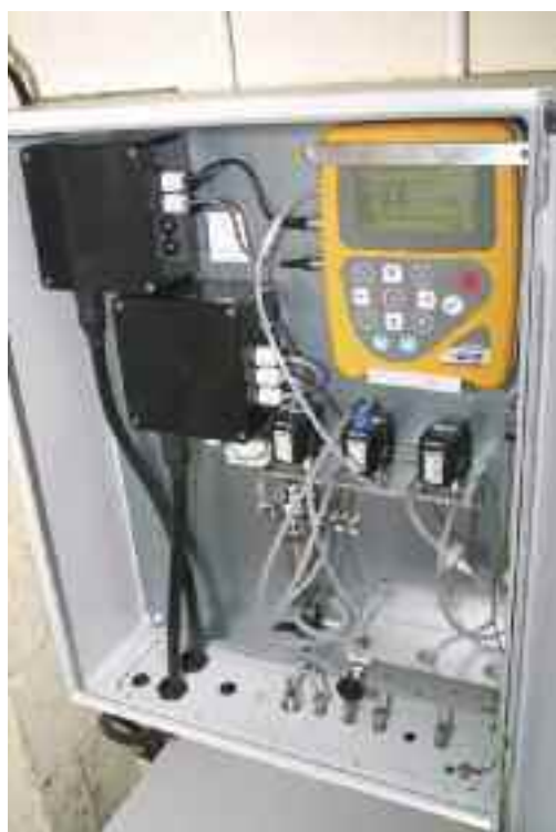
Remote and wireless static gas analyser is an Automatic Extraction Monitoring System, AEMS to auto-analyses gases including: CH 4 , H 2 S, O 2 , CO, CO 2 and auto-transmit secure data via the Internet.
