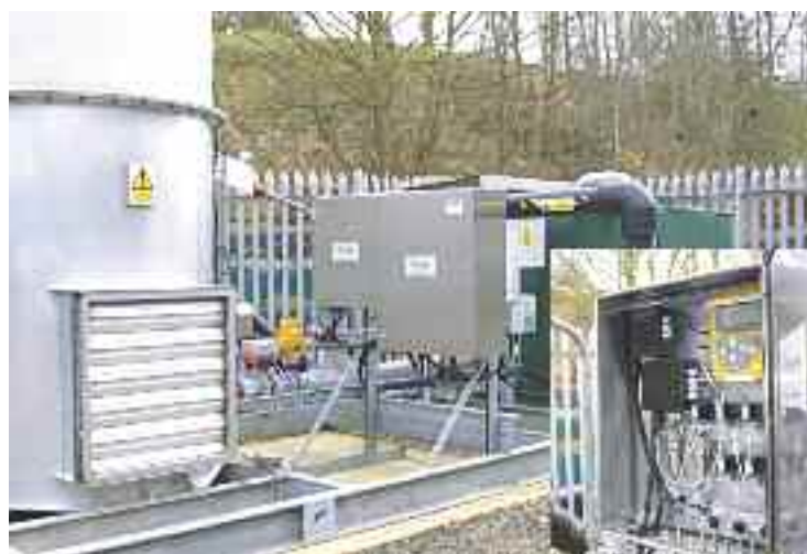
Extracted landfill gas for CHP or flaring is analysed, measured and monitored with data logged and securely transmitted to producers' Internet screens.
