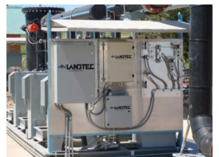
Automated landfill gas extraction monitoring system
