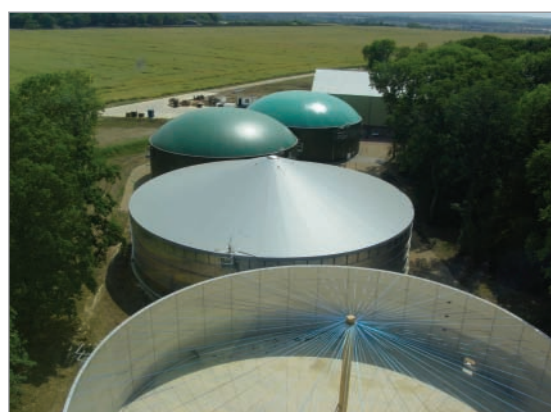
Anaerobic digesters at BiogenGreenfinch
