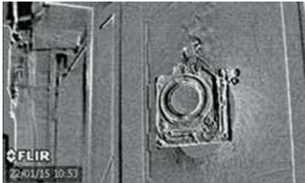
A FLIR GF306 can easily detect ammonia gases escaping from a gas nitriding furnace.
