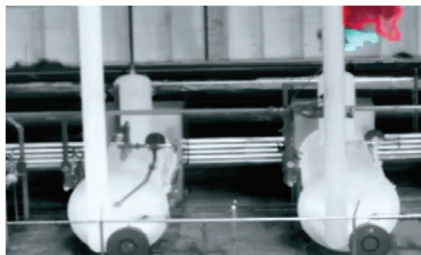
Alarming Leak (Area in Red)
