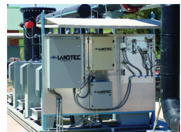
Unmanned Automatic Extraction Monitoring System (AEMS) Equipment
