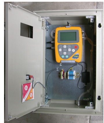
Field analytical unit - The remote gas analysis panel passes data to field server unit.
