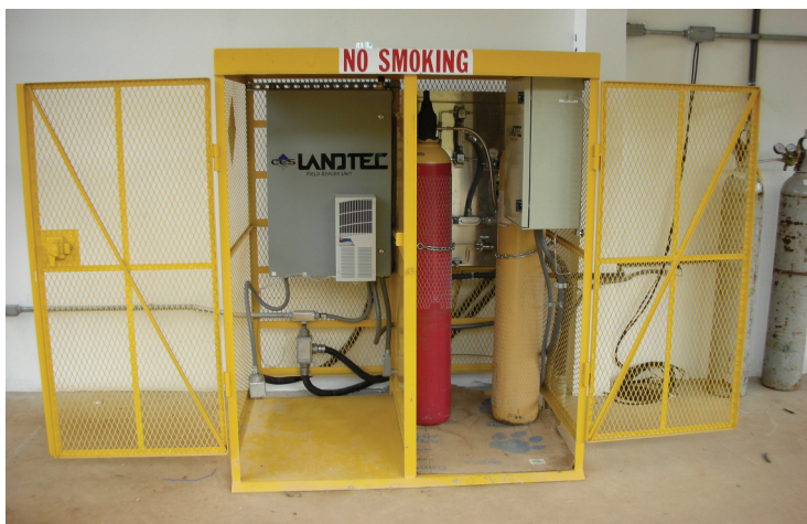
Automatic Extraction Monitoring Equipment in Brazil showing panels and gas bottles for calibration all in a security cage.
