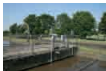
Fig. 2: Installation site of the NH4D sc ISE ammonium probe in the oxidation ditch
