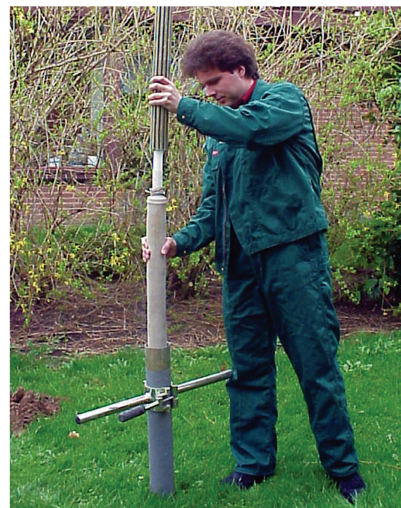
Installation of a Quality Well filterpack + bentonite collar in a bailer bored casing
