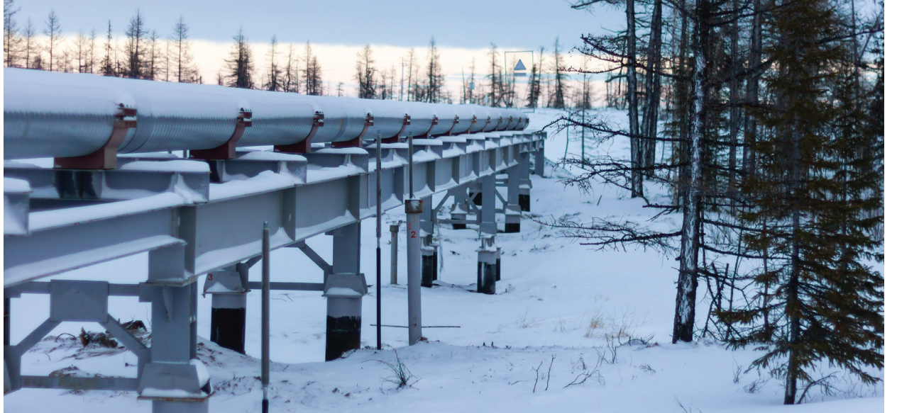
Gas pipeline through the wilderness
