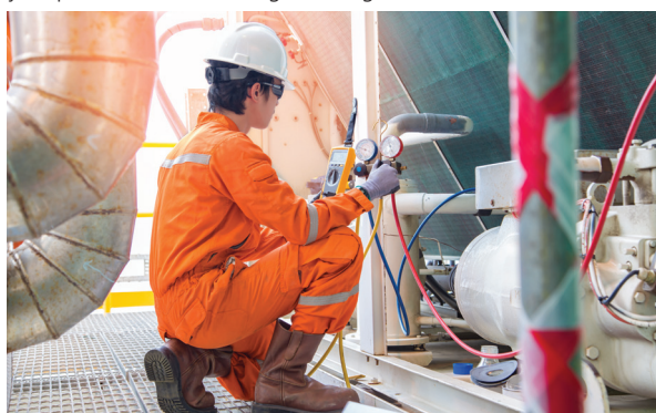
Gas detection on offshore gas rig
