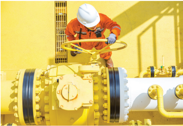
Gas pipeline valve
