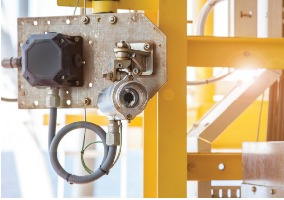
Line of sight gas detector on offshore rig
