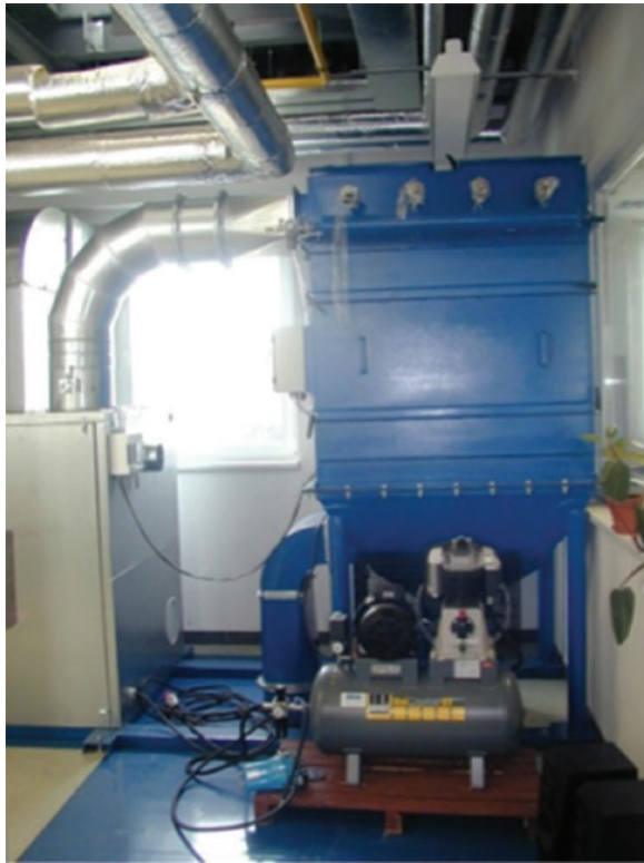
Fig 4. Covered exhausting fan on the left, filtration device on the right
