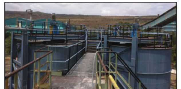
Figure 2. Four Carbonation tanks at Tummalapalle Mill.
