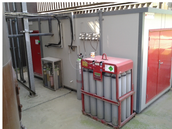
The cabin housing the AMS instruments with the sample extraction line and gas supply systems.
