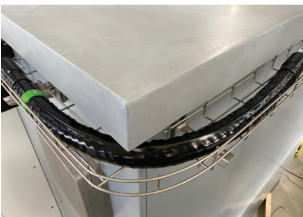
Extruded Flex in Cable Tray and Analyser Container
